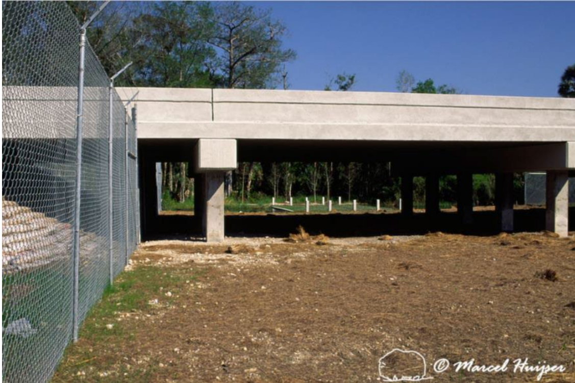
Figure 52: Wildlife underpass for Florida panthers ( Puma concolor coryi ), about 119 ft (36 m) wide (but only 21-26 m wide at grade level) and about 10-13 ft (3-4 m) high, just after construction in 1998, SR 29, Florida, USA.
