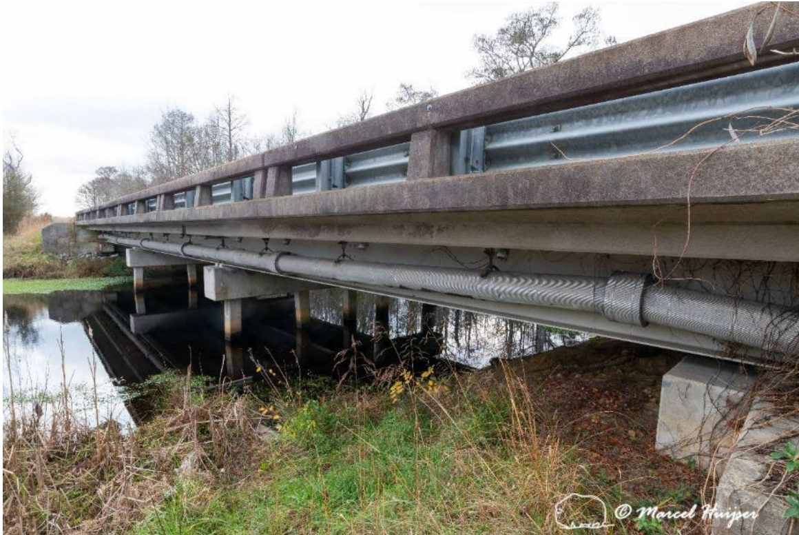
Figure 72: Hwy 94, Bridge across Riders Creek, north of junction with Frying Pan Rd., North Carolina.
