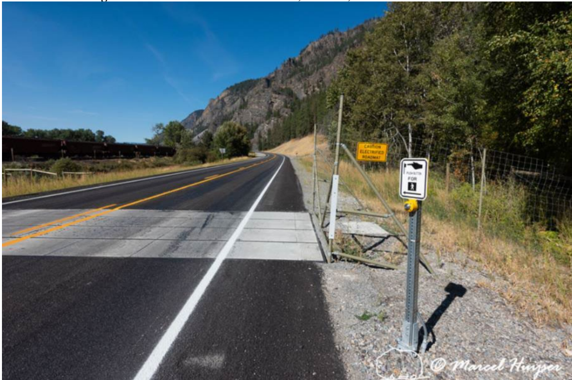
Figure 44. Electrified barrier embedded in travel lanes to keep large mammals, including bighorn sheep, out of fenced road corridor, MT Hwy 200, Thompson Falls, Montana, USA.
