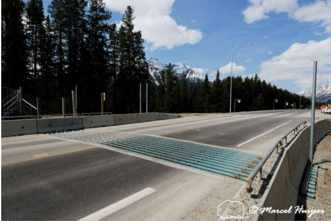
Figure 43. Fence-end brought close to the edge of the pavement, protected by Jersey barriers. Also note that there is a wildlife guard embedded in the travel lanes, Alberta, Canada.
