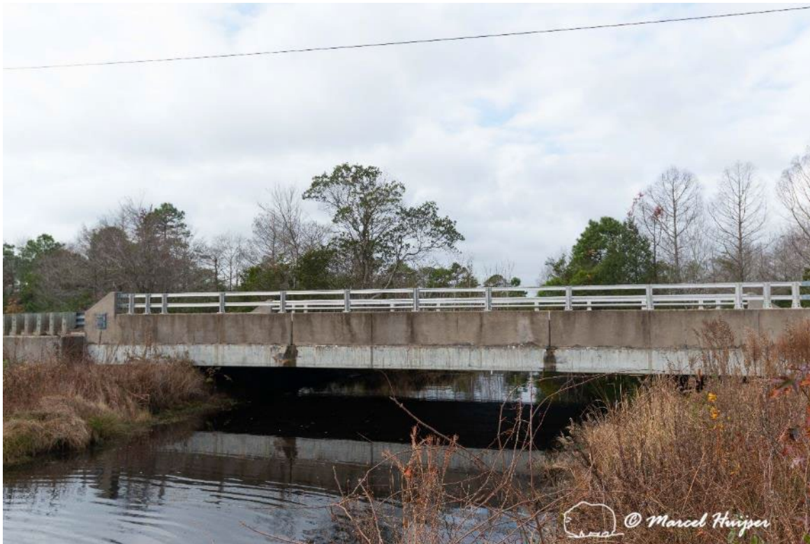
Figure 64: US Hwy 264, bridge at Point Peter Rd, Alligator River NWR, North Carolina.
