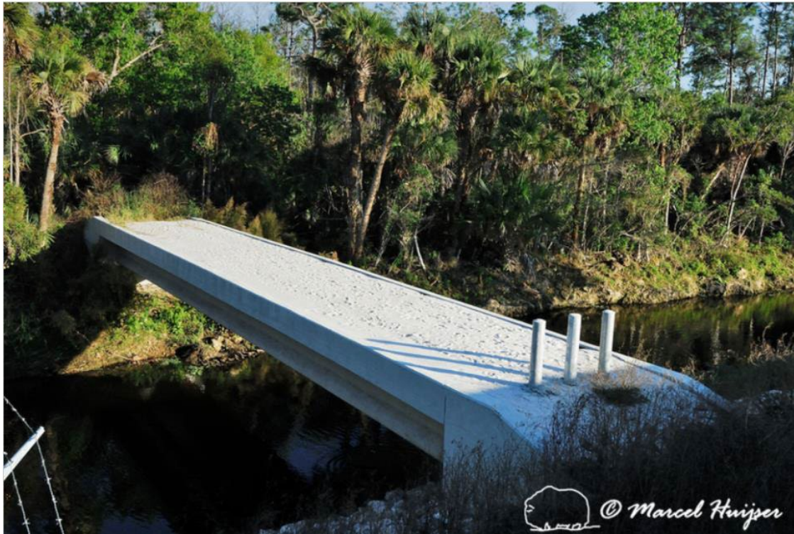
Figure 54: Wildlife underpass for Florida panthers ( Puma concolor coryi ) (to the right, outside of image) and a wildlife bridge across canal, SR 29, Florida, USA. Note that the posts on the bridge block illegal use of motorized vehicles such as ATVs.
