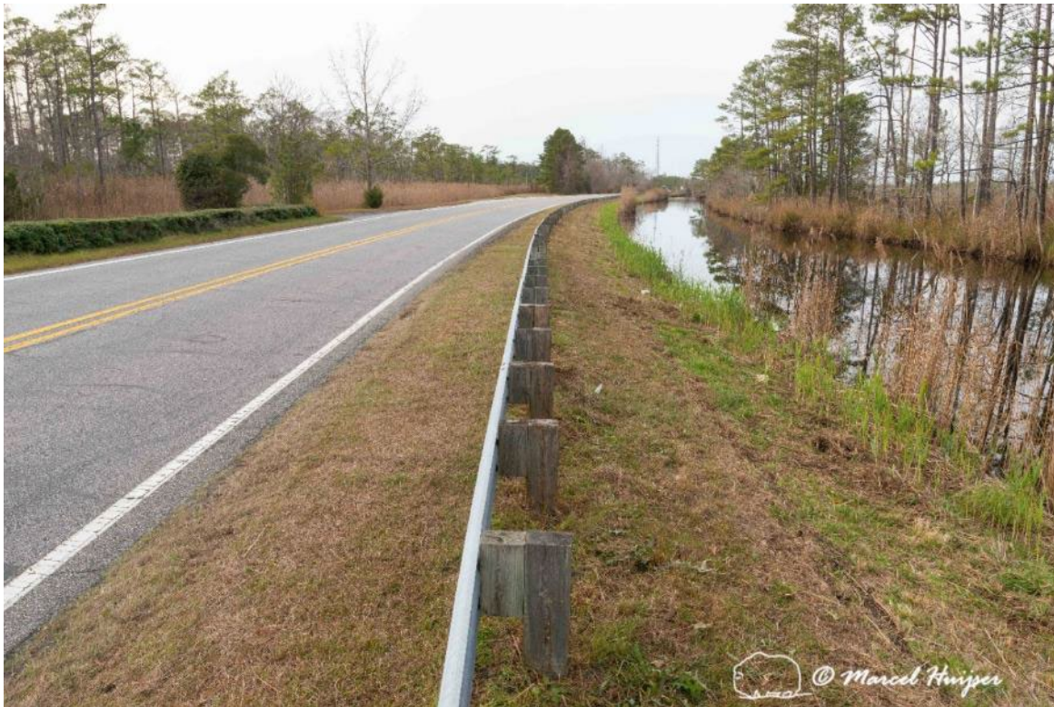
Figure 58: US Hwy 64 and adjacent canal at Milltail Rd, Alligator River National Wildlife Refuge, North Carolina.
