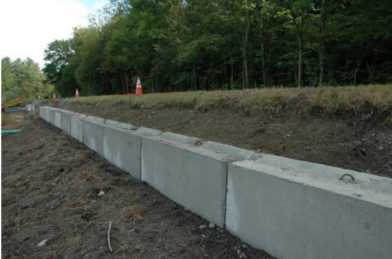
Figure 3: Installation (top) and completion (bottom) of a barrier wall for amphibians made from concrete waste blocks on Monkton Road, Vermont. Photo Credit: Chris Slesar, Monkton Conservation Commission.
