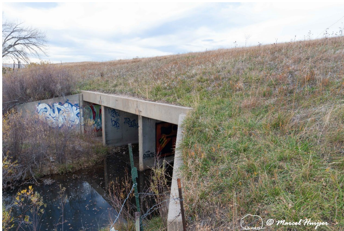
Figure 22: Divided box culvert, Coal Creek (Hwy 128, mile reference post 0.47), south side, inflow.
