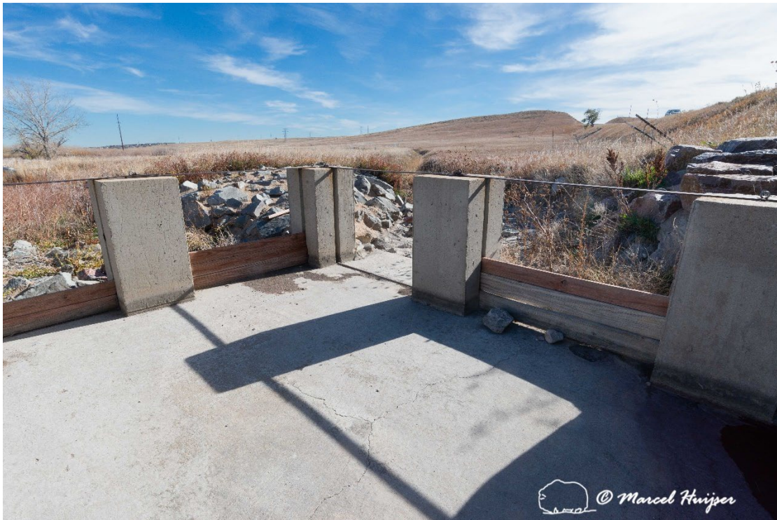
Figure 28: Outflow structures, Walnut Creek (Indiana St., 0.62 mile south of junction with Hwy 128), east side, outflow.
