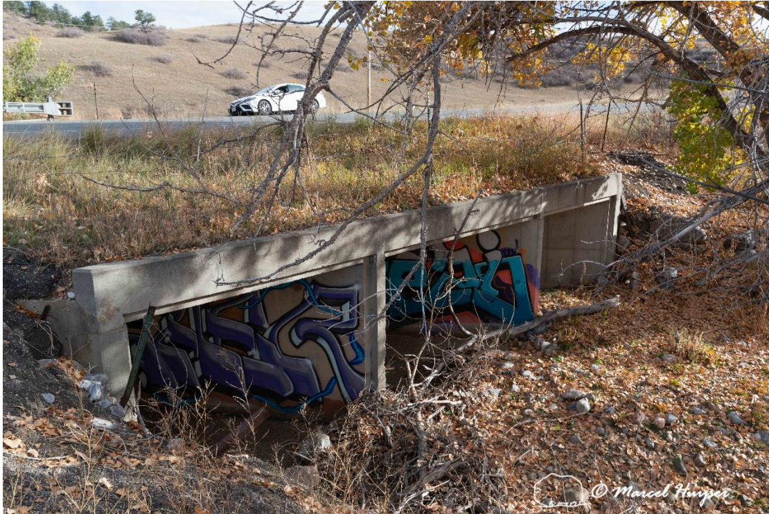
Figure 20: Divided box culvert, Coal Creek (Hwy 93, mile reference post 10.95), west side, inflow.
