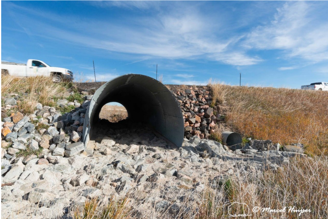
Figure 30: Riprap at inflow, South Woman Creek (Indiana St., 2.25 mile south of junction with Hwy 128), west side, inflow.
