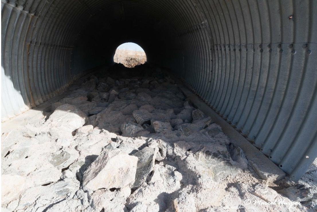
Figure 31: Riprap inside culvert, South Woman Creek (Indiana St., 2.25 mile south of junction with Hwy 128), west side, inflow.
