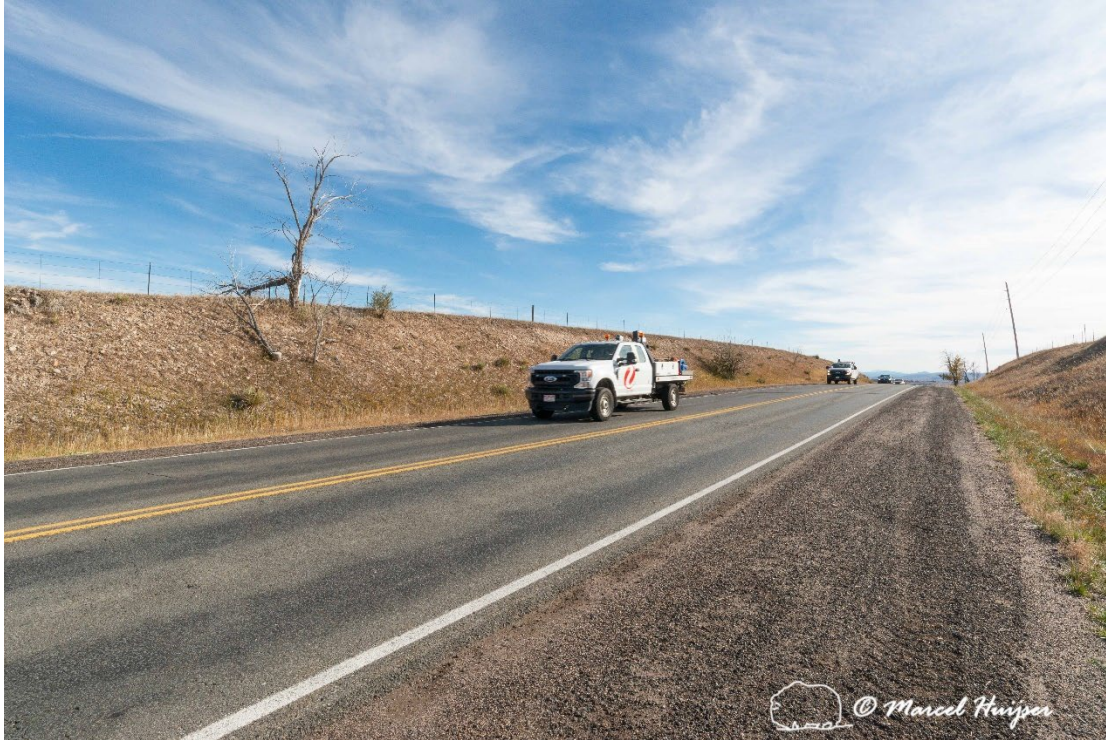
Figure 49. The roadcut along Indiana St., about 1.3 miles south of the junction with Hwy 128.
