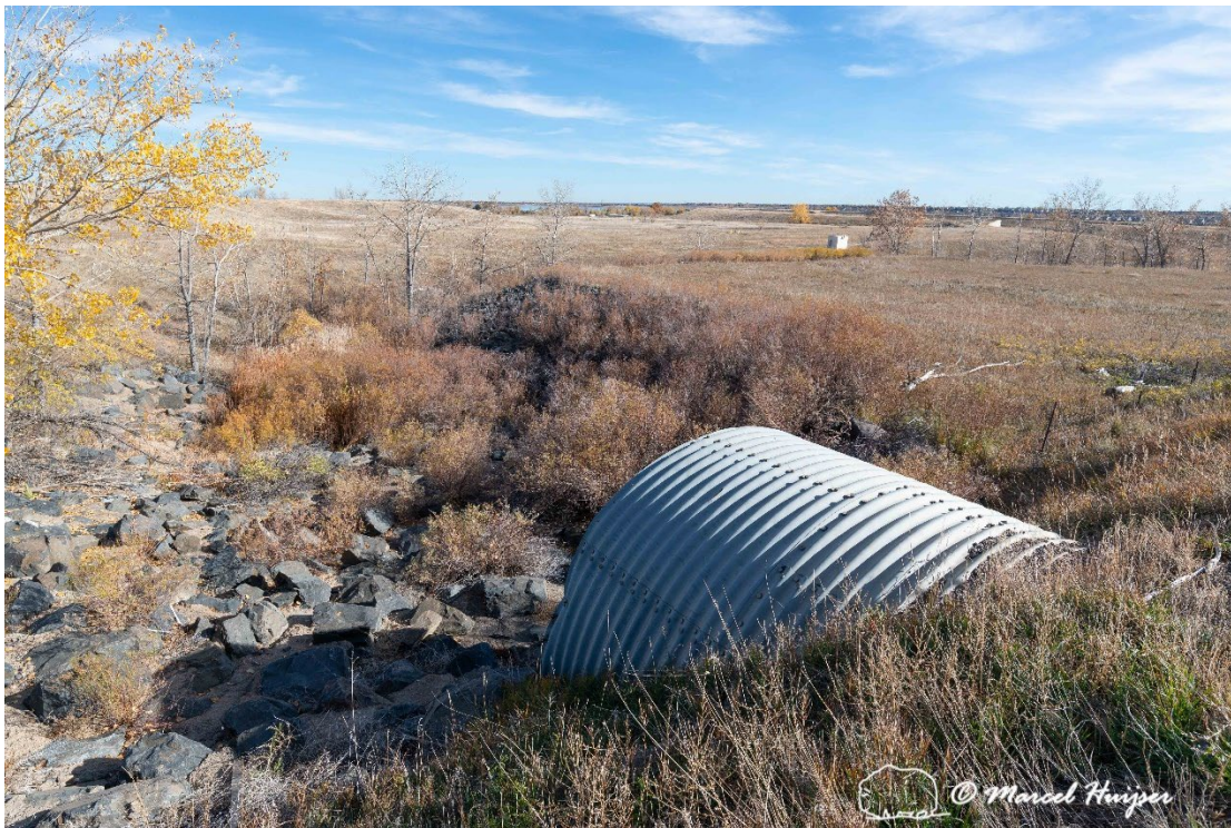
Figure 32: Riprap at outflow, South Woman Creek (Indiana St., 2.25 mile south of junction with Hwy 128), east side, outflow.
