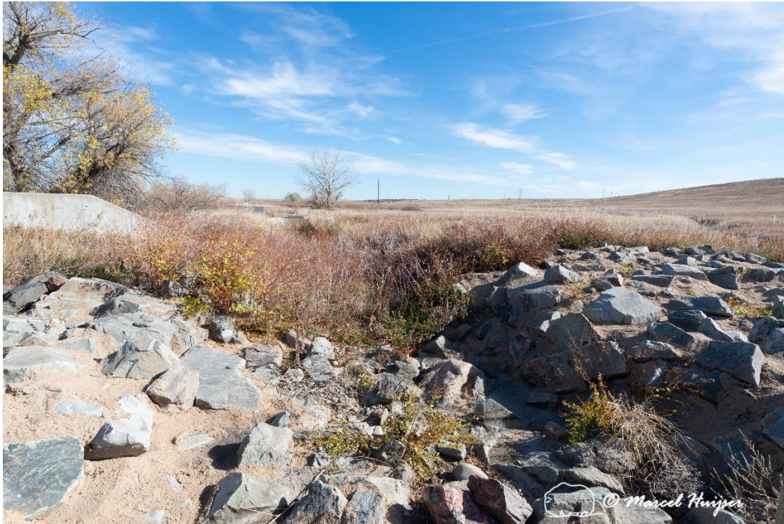
Figure 29: Riprap at outflow, Walnut Creek (Indiana St., 0.62 mile south of junction with Hwy 128), east side, outflow.
