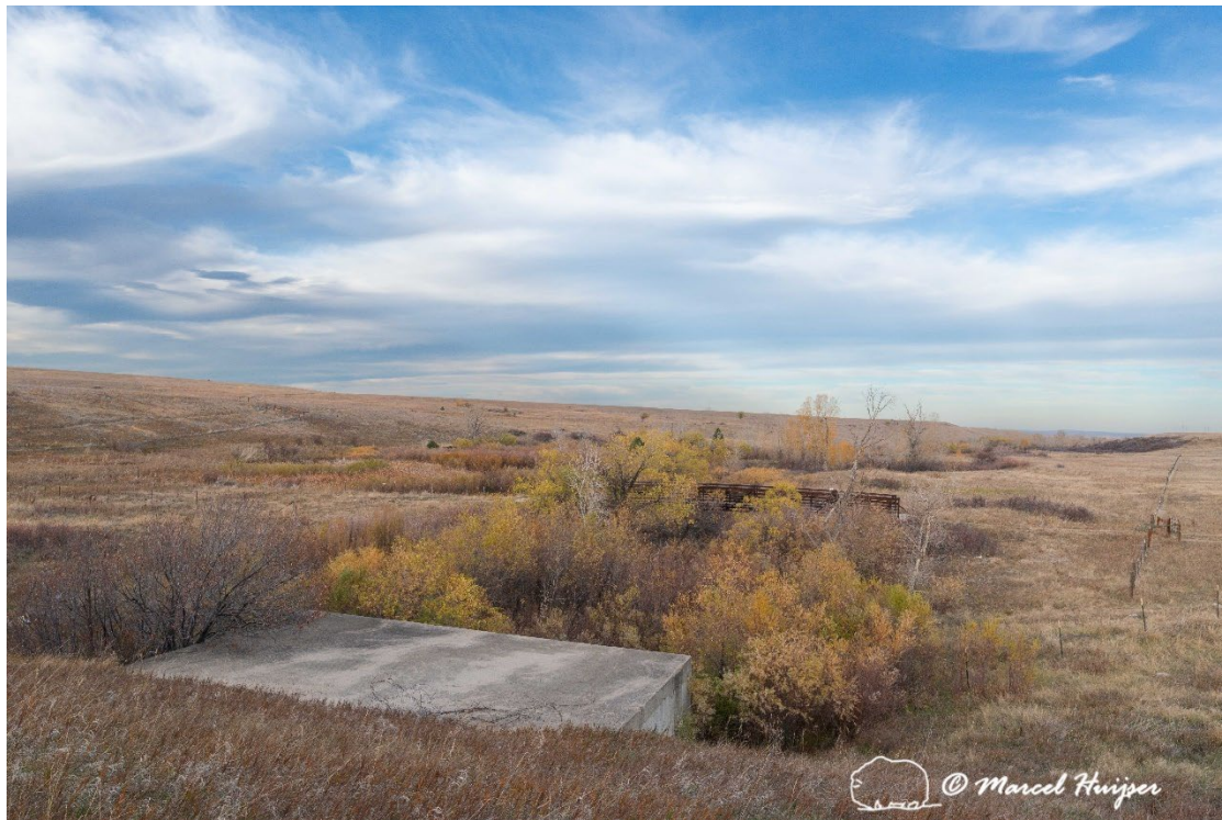
Figure 23: Divided box culvert, Coal Creek (Hwy 128, mile reference post 0.47), north side, outflow.
