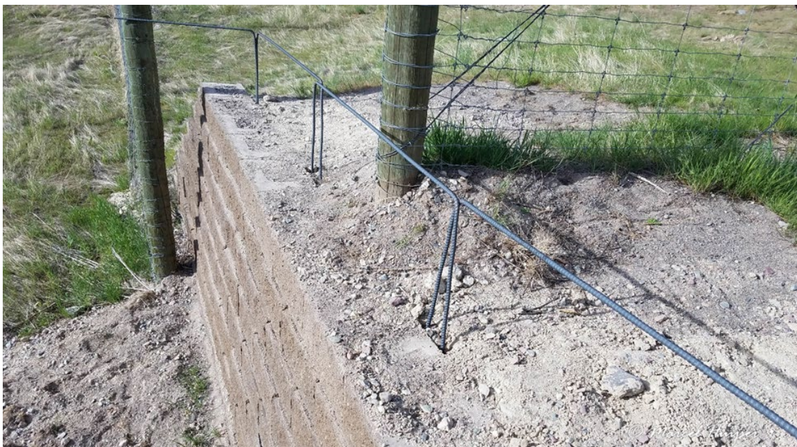
Figure 11: The rebar had a minimum setback of 30 cm (12 inches) as the legs had to be positioned behind the concrete blocks of the face of the jump-out.
