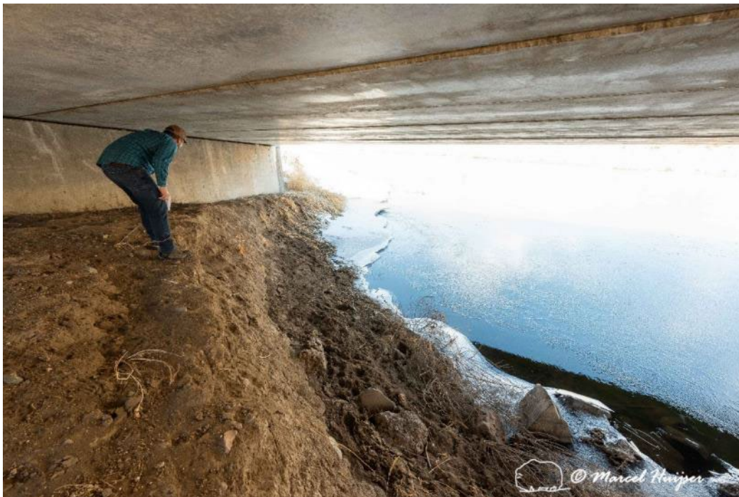
Figure 48. An eroded slope can reduce use of an underpass by large wild mammals.
