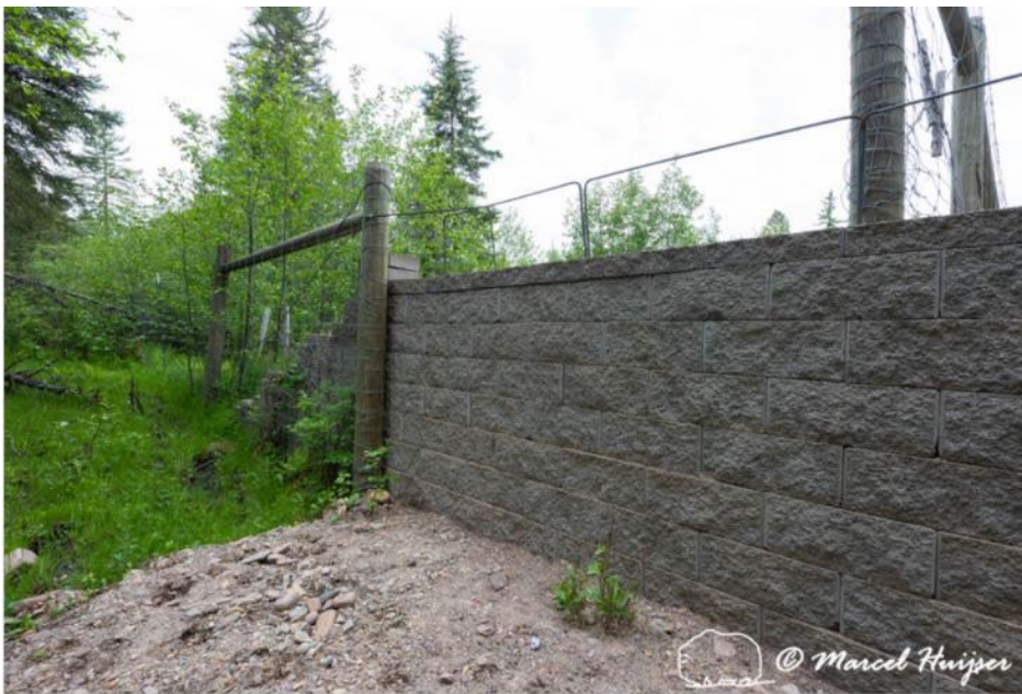
Figure 28. Wildlife jump-out along US Hwy 93, Flathead Indian Reservation, Montana, USA. Jump out is 5 ft tall with rebar on top.
