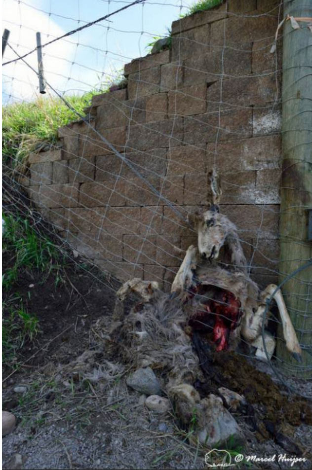
Figure 7. Mule deer got stuck between wildlife fence and the wing wall associated with a wildlife underpass and died, Montana, USA. The fence should be snug up to the wing wall. Here the last fence post was close enough to the wing wall but the second to last post allowed for a funnel or wedge like configuration making the deer believe it could potentially pass in between the wall and the fence. When it realized it could not go forward anymore it tried to turn itself around and then got stuck and died. It is important that both the post and the fence are positioned such that no space is left between the wing wall and the fence.
