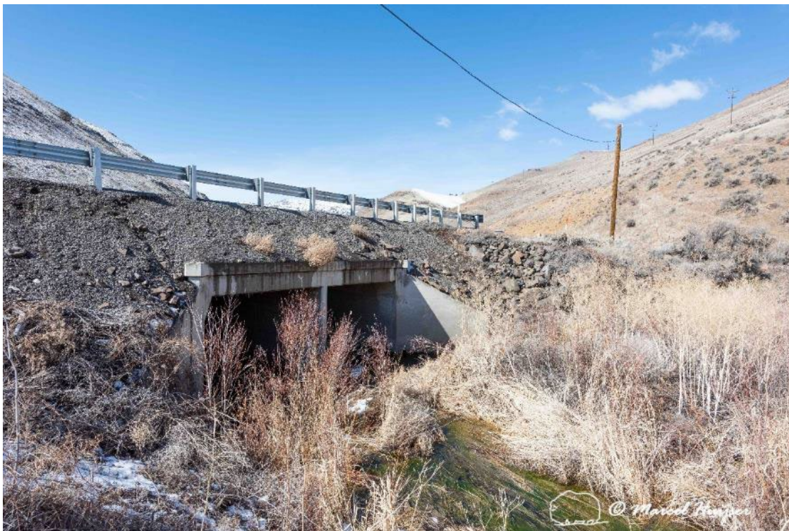
Figure 46. A double box culvert like this one is likely too small for mule deer (width and height).
