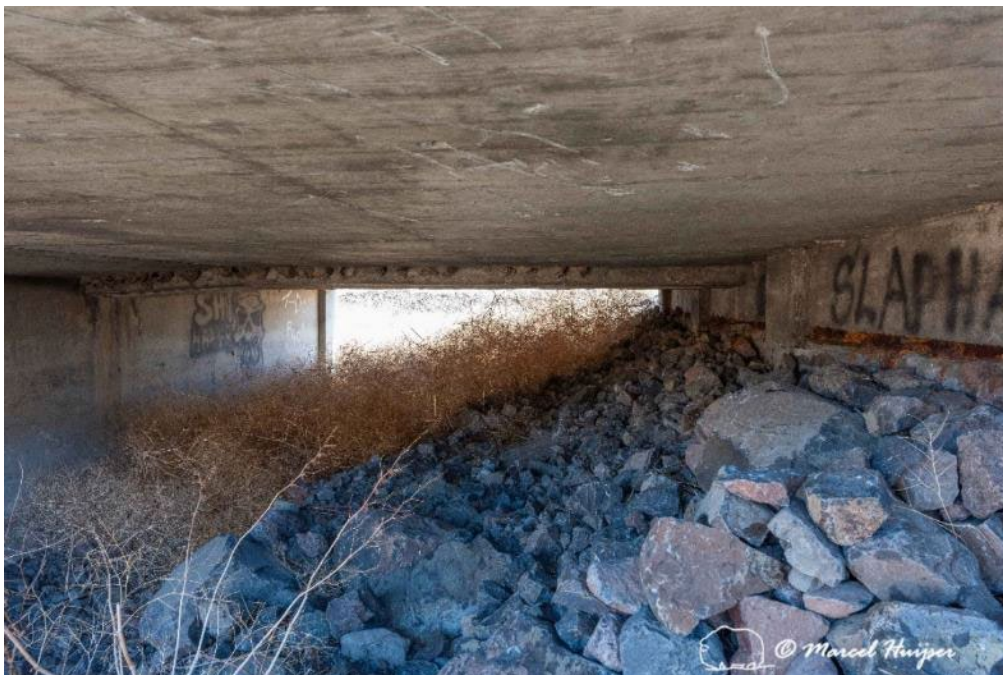
Figure 44. Riprap (large rocks and boulders) and tumble weed that has accumulated inside a structure or on its approaches can be a physical barrier to mule deer and other large ungulates.
