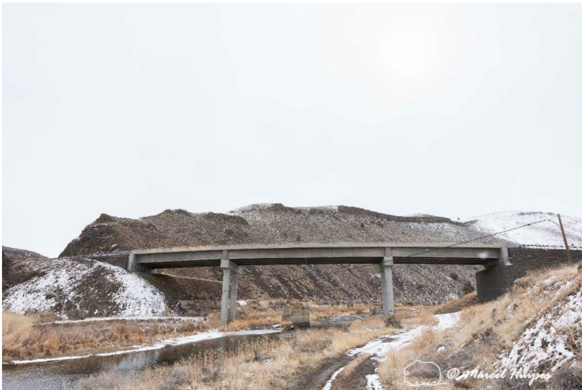
Figure 42. This bridge is sufficiently wide and high for mule deer, it has a good line-of-sight through the structure, and there is enough dry and flat terrain for them to travel under the bridge, at least in winter.
