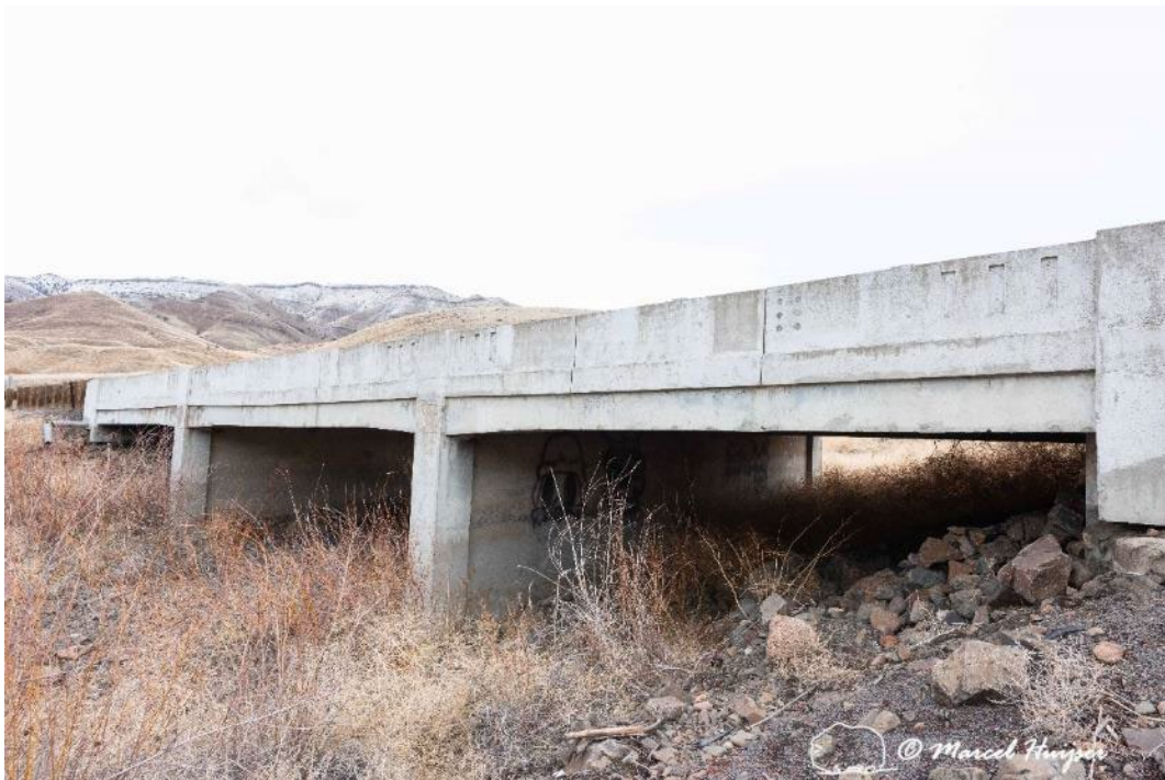
Figure 51. A structure with walls typically hinders visibility under the bridge and hinders a good line-of-sight towards the other side of the road.
